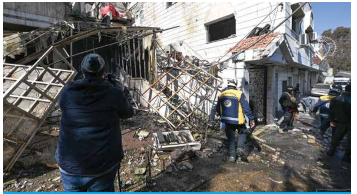
DAMASCUS: Syrian White Helmets rescuers inspect the site of a Zionist air strike on a building in Damascus.
