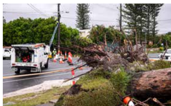
SYDNEY: Workers fix electricity wires next to a tree uprooted by strong winds from Cyclone Alfred in the suburb of Eianora on the Gold Coast on March 8, 2025. — AFP
