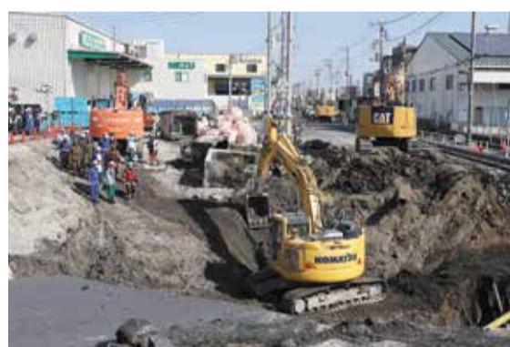
YASHIO: Excavators and rescue personnel working to construct a slope for rescue operations are seen at the site where a truck plunged into a sinkhole, trapping the vehicle's driver, in Yashio, Saitama Prefecture. — AFP
