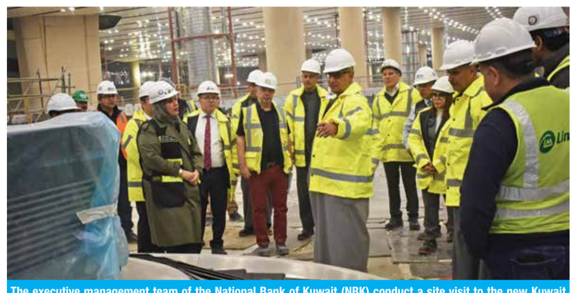
The executive management team of the National Bank of Kuwait (NBK) conduct a site visit to the new Kuwait Airport terminal project (T2).
