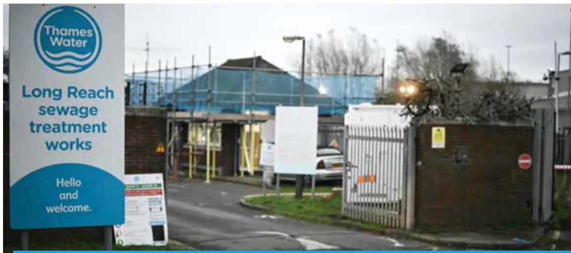
DARTFORD: A photograph shows a board sign with the logo of the company at the entrance of Thames Water's Long Reach Sewage Treatment Plant, in Dartford, east of London. — AFP
