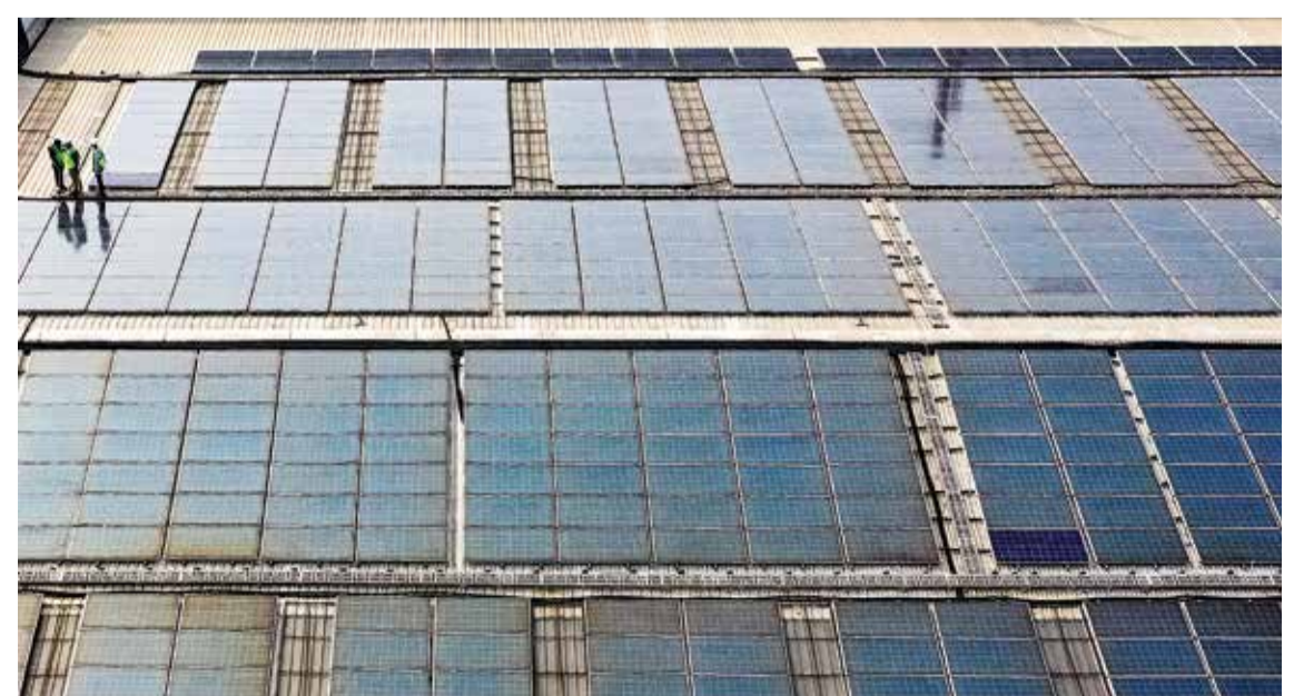
GREATER NOIDA: Photo shows an aerial view of solar panels installed by SunSource Energy at a food processing plant in Greater Noida. — AFP
