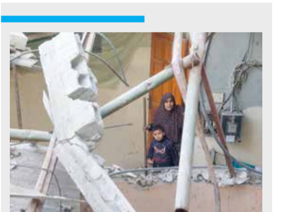
GAZA: A Palestinian woman and a child stand at the door of a house next to a building destroyed in a Zionist strike in the Nuseirat camp in central Gaza on Dec 10, 2024. — AFP
