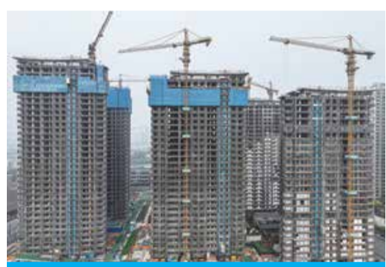
An aerial view of residential buildings under construction in Nanjing, in eastern China's Jiangsu province. — AFP
