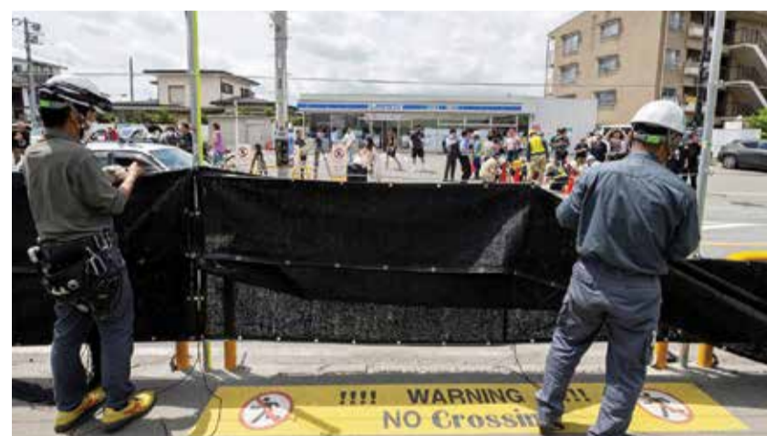
Workers install a barrier to block the sight of Japan's Mount Fuji emerging from behind a convenience store to deter badly behaved tourists, in the town of Fujikawaguchiko, Yamanashi prefecture. — AFP photos
