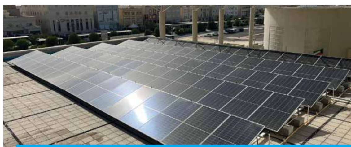
Smart school rooftop solar panels to reduce pressure on electricity.
