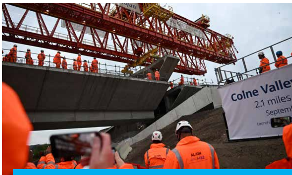
Workers look at the final deck segment of HS2's 2.1-mile as it is fixed on the viaduct crossing the Colne Valley, in Maple Cross, north-west of London, on Sept 5, 2024. — AFP
