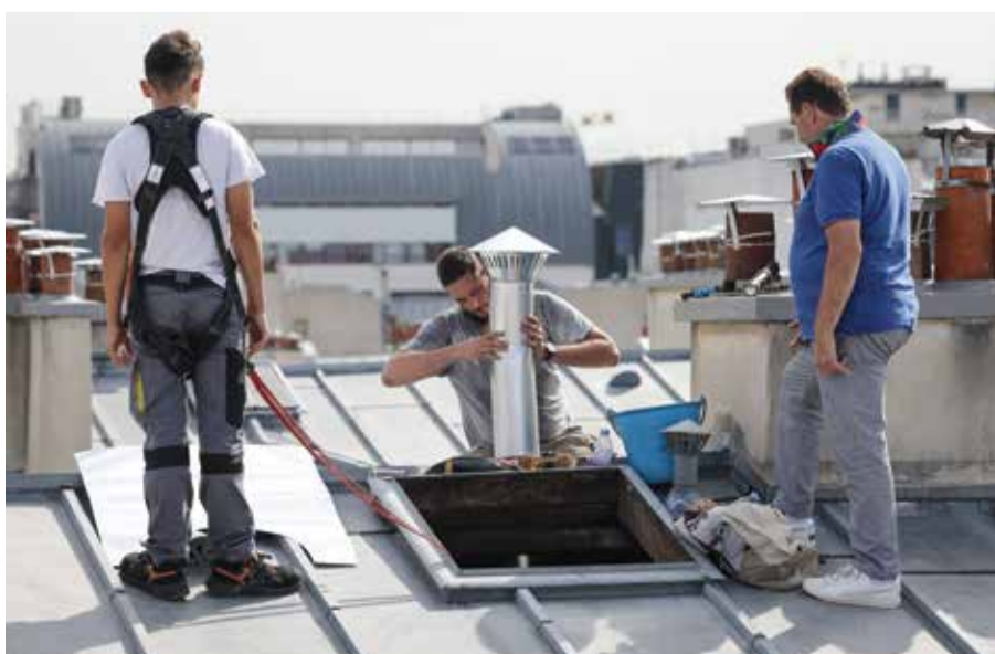
Romain Florentin (center) flanked by Thierry Gesset-Parment, business manager of ATZ - L'Art du Toit company and president of CAPEB Grand Paris (right), and his apprentice (left), works on the roof of a building in Paris.
