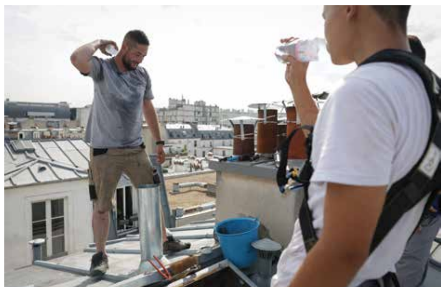
Romain Florentin (left) and his apprentice, cool off as they work on the roof of a building in Paris.
