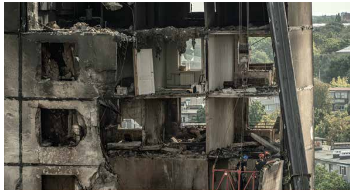
KHARKIV: Ukrainian emergency workers inspect a heavily damaged residential building following a recent missile attack in Kharkiv, on August 31, 2024. — AFP
