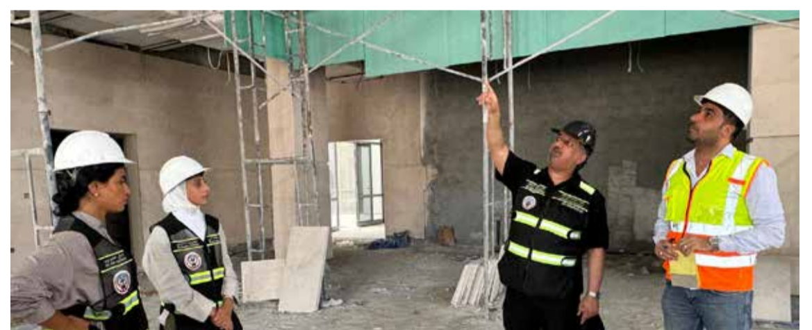
KUWAIT: Assistant Undersecretary for Engineering Affairs and Projects Ibrahim Al-Naham and specialized engineering teams inspect the Abdulrahman and Waleed Manahi Al-Asimi Cardiac Intensive Care Center. — KUNA photos
