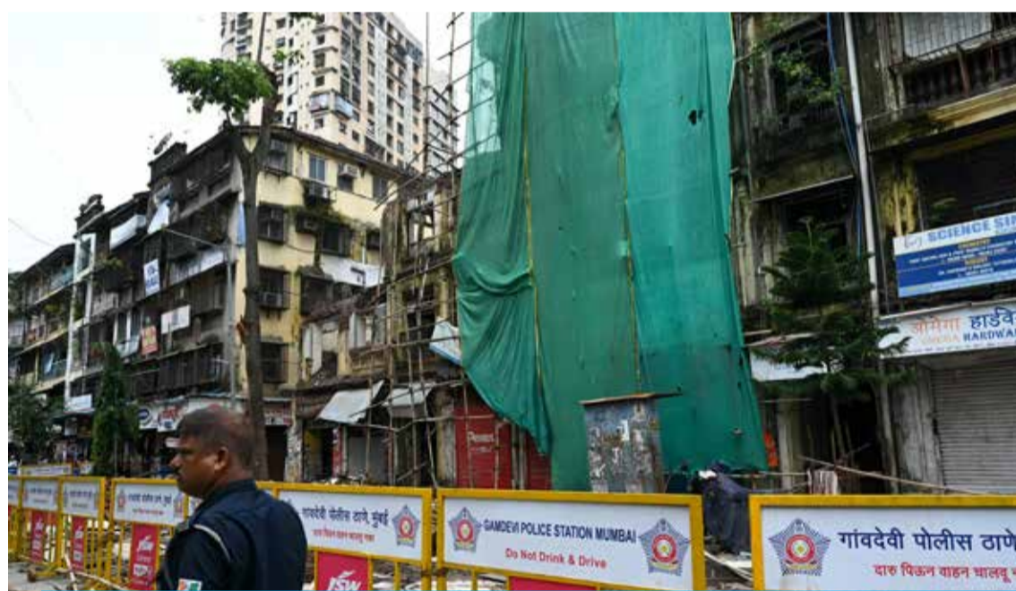
MUMBAI: A security guard stands outside the Rubbunnisa Manzil building, partially collapsed after monsoon rains in Mumbai. - AFP
