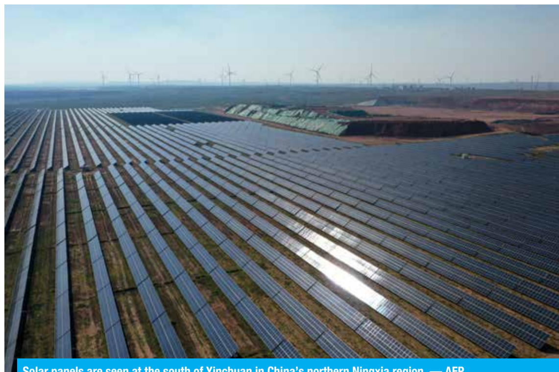
Solar panels are seen at the south of Yinchuan in China's northern Ningxia region. — AFP
