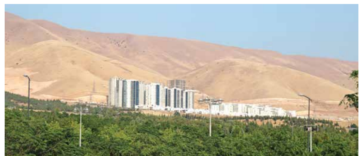
Buildings under construction at the site of a real estate project in Sulaimaniyah.
