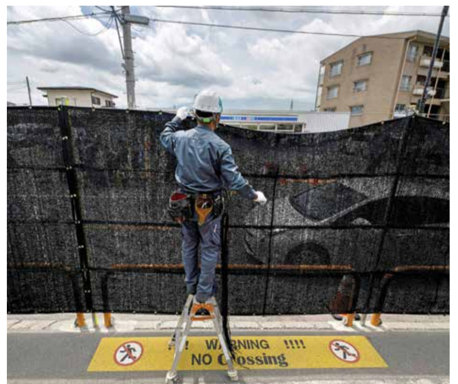
This photo taken on May 21, 2024 shows a worker installing a barrier to block the sight of Japan's Mount Fuji emerging from behind a convenience store to deter badly behaved tourists, in the town of Fujikawaguchiko, Yamanashi prefecture. - AFP
