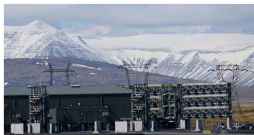
The new plant of Swiss start-up Climeworks is pictured in Hellisheidi, Iceland on May 8, 2024. — AFP
