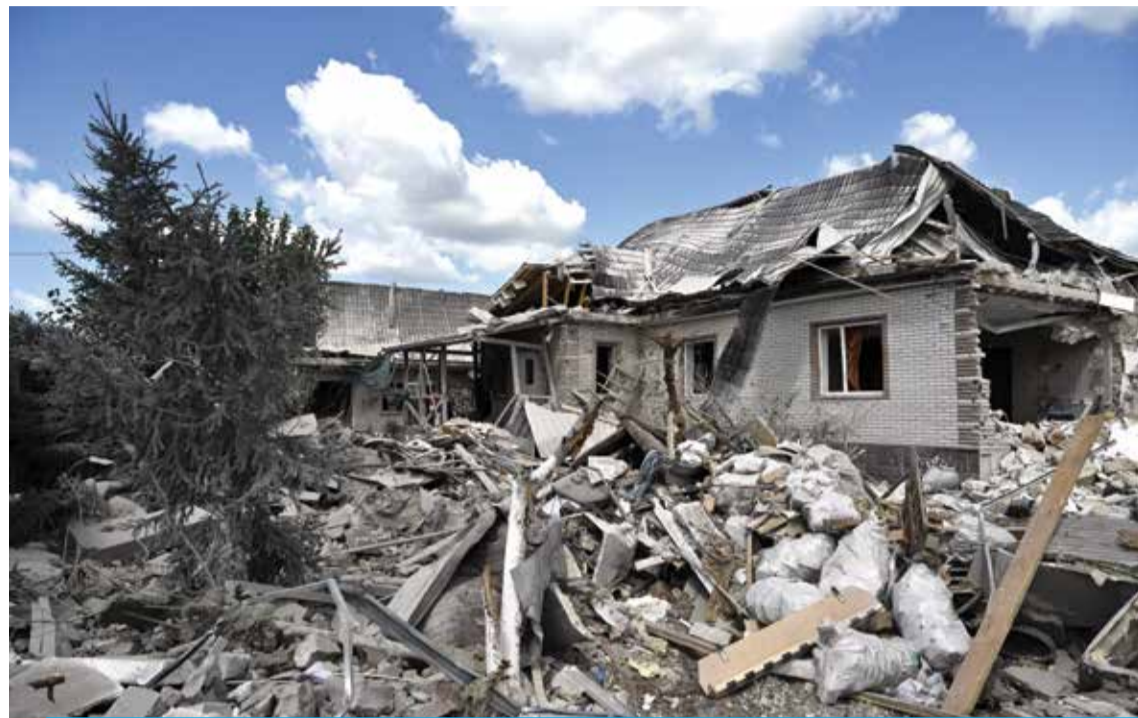
KYIV: This photograph shows a residential house, heavily damaged following a Russian missile strike on August 11, 2024, in a village in the Brovary district, Kyiv region. — AFP photos
