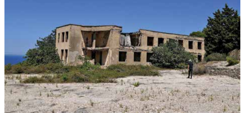
An abandoned ex-military command building on a hilltop on the island of Sazan, near the Albanian city of Vlora, on Mediterranean coast. — AFP photos
