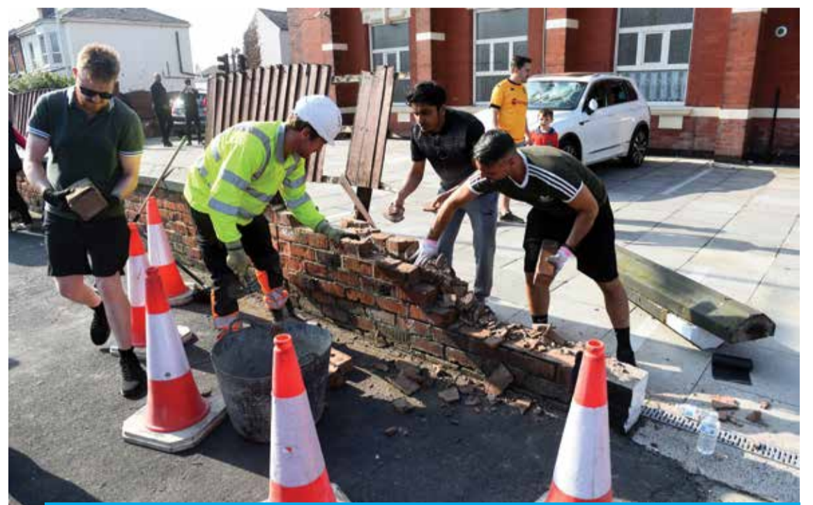
SOUTHPORT: Volunteers help repair damage done to the Southport Islamic Society Mosque in Southport, northwest England, on July 31, 2024 following clashes after a deadly knife attack. — AFP
