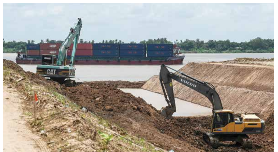
PREK TAKEO: A ship transports containers along the Mekong River (back) as excavators are used to dig the Funan Techo canal along the Prek Takeo channel in Kandal province. — AFP
