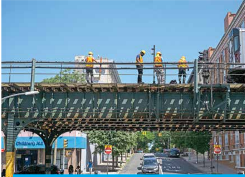
NEW YORK: Workers repair a subway train platform during a summer heat wave in the Bronx borough of New York on July 11, 2024. — AFP photos
