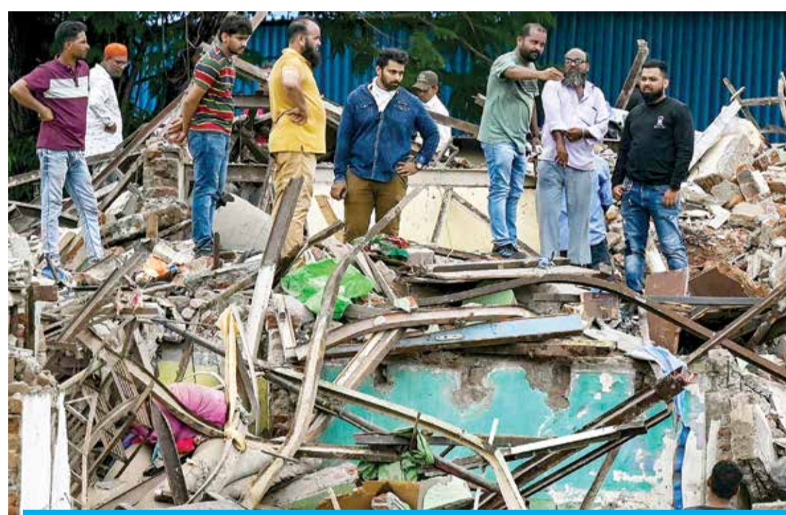
MUMBAI: Residents stand amid the debris of their allegedly illegal houses demolished by civic authorities in Mumbai. — AFP
