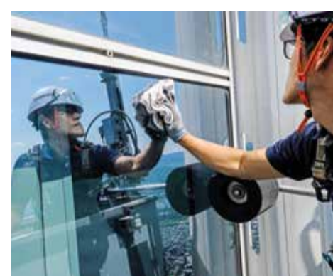
In this photo Seo Seung-ho cleans a window with a cloth coated with diatomaceous earth as he stands on a special "gondola" suspended by cables from the 125th floor of the building in Seoul.
