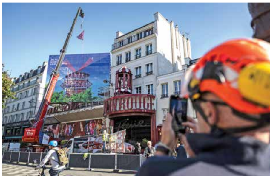
A passerby takes a picture of a crane lifting one of the four temporary windmill sails during its installation on the top of the Moulin Rouge cabaret following the collapse of the former ones, in Paris.
