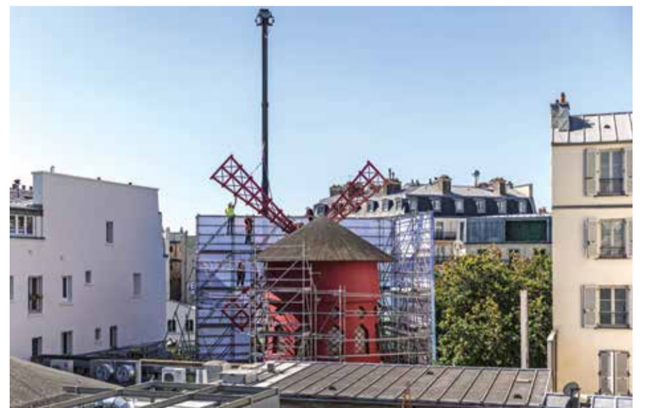
Workers install one of the four temporary windmill sails on the top of the Moulin Rouge cabaret following the collapse of the former ones, in Paris. — AFP photos
