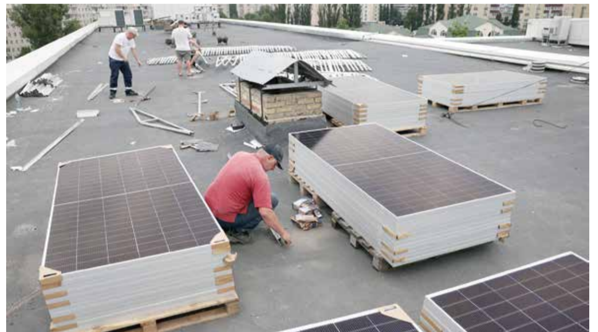
KYIV: Workers install solar panels on the roof of Maternity House No 3 during a partial electricity blackout in Kyiv on June 14, 2024, following Russian strikes on Ukrainian energy infrastructure. — AFP
