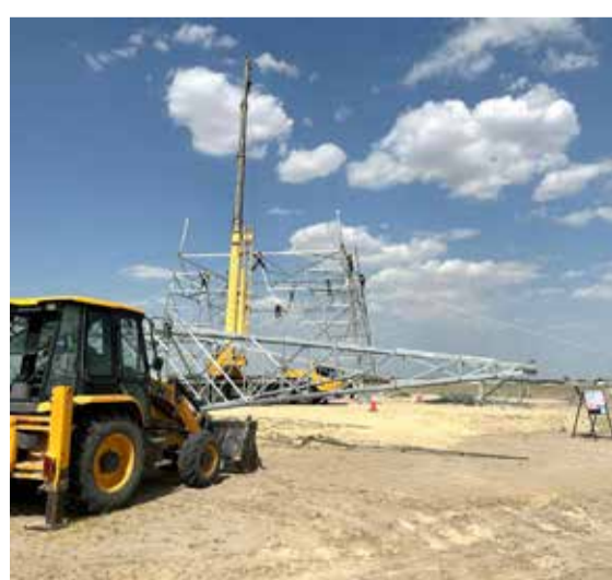
KUWAIT: A worksite, part of the Gulf electrical interconnection expansion project, is seen in this photo.
