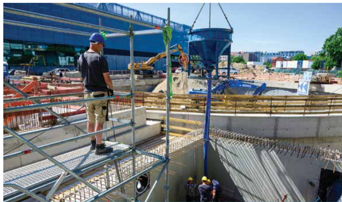
BERLIN: A cement container is lowered into a construction site during work on a 17,000 m3 underground rainwater overflow basin for the Berliner Wasserbetriebe (Berlin waterworks), in Berlin's Mitte district on May 17, 2024. — AFP
