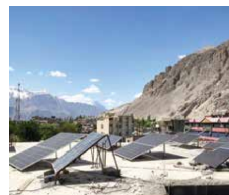
This photograph shows solar panels installed on the roof of a building in Skardu.
