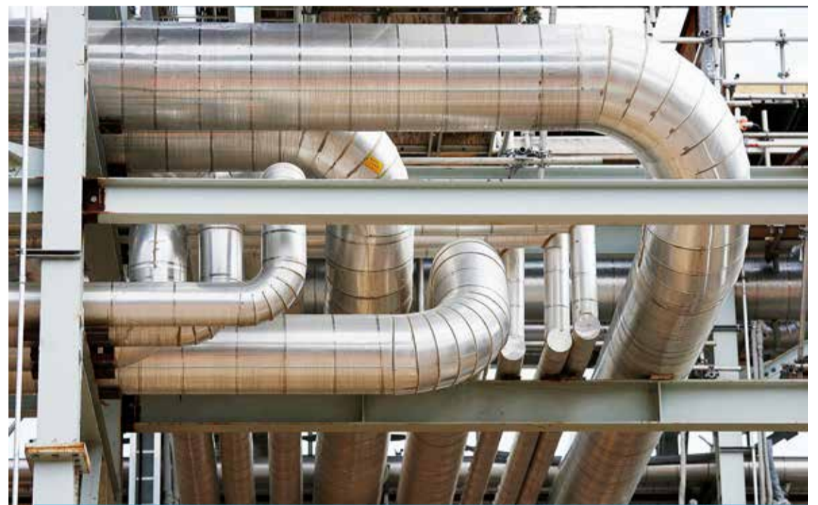
A view of oil production pipes at the Cenovus Foster Creek SAGD oil sands operations near Cold Lake, Alberta, July 9, 2012. — Reuters
