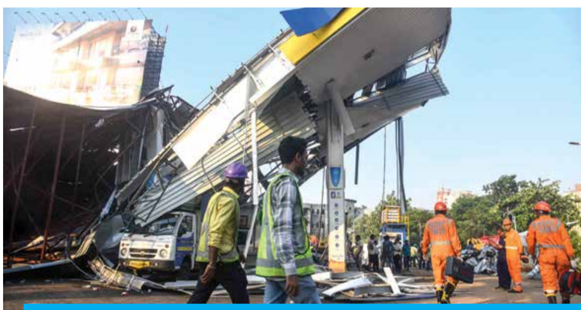
MUMBAI: National Disaster Response Force (NDRF) personnel (right) and rescue workers inspect the site a day after an advertisement billboard collapsed at a petrol station following a storm, in Mumbai on May 14, 2024. — AFP
