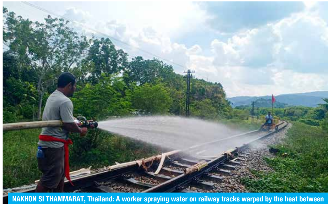
NAKHON SI THAMMARAT, Thailand: A worker spraying water on railway tracks warped by the heat between Ron Phibun district and Khao Chum in the southern Thai province of Nakhon Si Thammarat.
