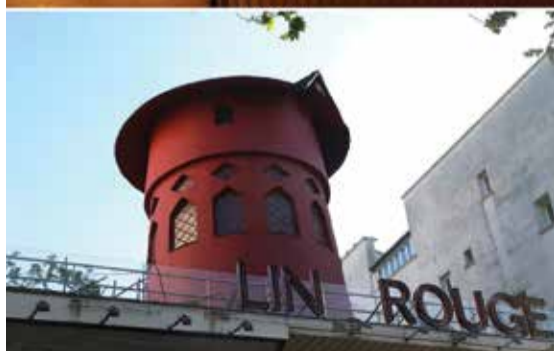
This combination of pictures created on April 25, 2024, shows the Moulin Rouge, a famous cabaret and theatre at night in Paris, on October 13, 2023, and the cabaret mill without the blades and part of the missing sign, after the Moulin Rouge windmill collapsed during the night without causing any injuries, firefighters told AFP, in Paris, on Thursday. — AFP
