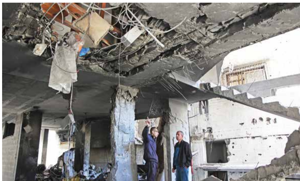
GAZA: Palestinians inspect the damage to the home of the Tabatibi family after Zionist bombardment in the Daraj neighborhood of Gaza on April 12, 2024. — AFP
