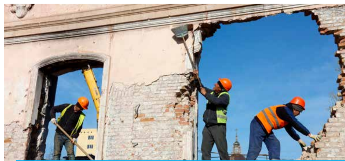
MARIUPOL: Construction workers clean the wall of a house to be restored in Mariupol, Russian-controlled Ukraine. — AFP
