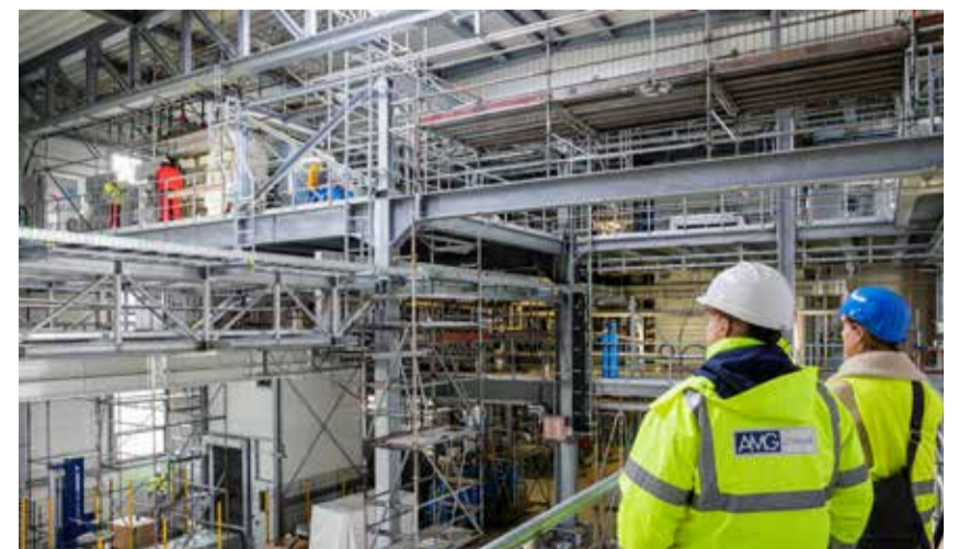
BITTERFELD-WOLFEN, Germany: The construction site of AMG Lithium GmbH, a subsidiary based in Germany and part of the AMG Clean Energy Materials division of AMG Critical Materials NV at the Bitterfeld site in Bitterfeld-Wolfen, eastern Germany. — AFP
