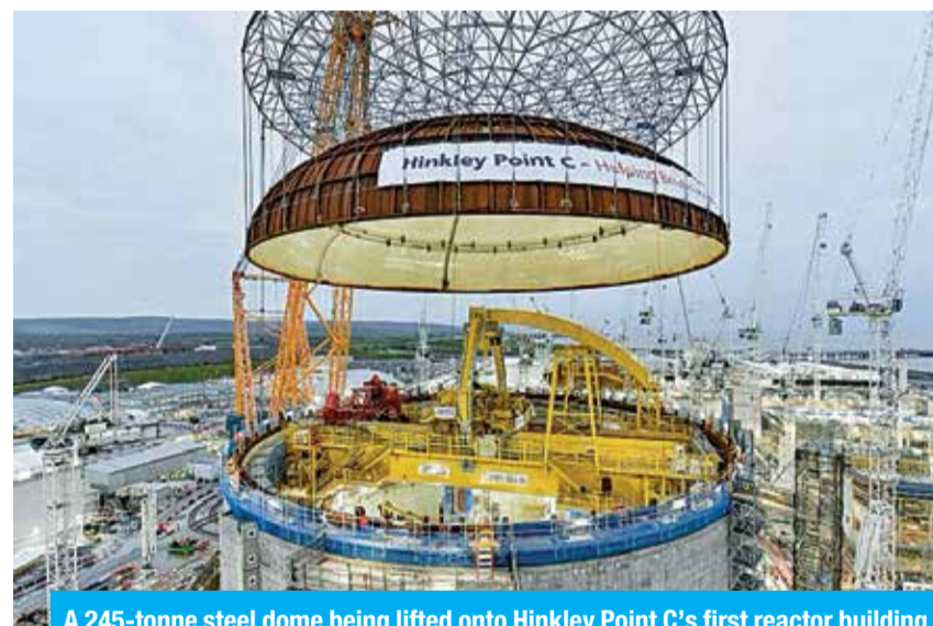
A 245-tonne steel dome being lifted onto Hinkley Point C's first reactor building near Bridgwater in south-west England on Dec 15. — AFP
