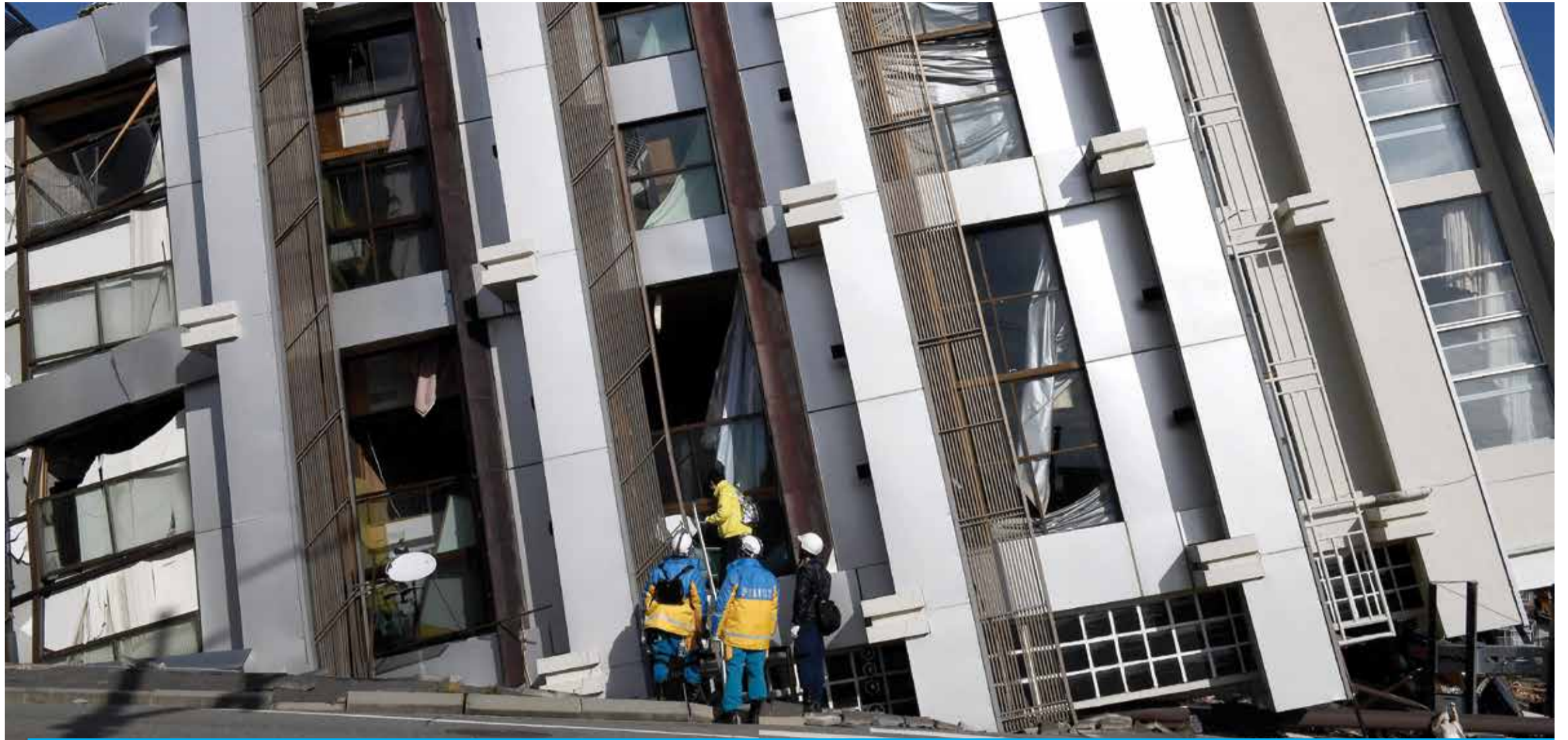
WAJIMA: Police officers check a collapsed building in the city of Wajima, Ishikawa prefecture, on Jan 5, 2024, after a major 7.5 magnitude earthquake struck the Noto region on New Year's Day. — AFP
