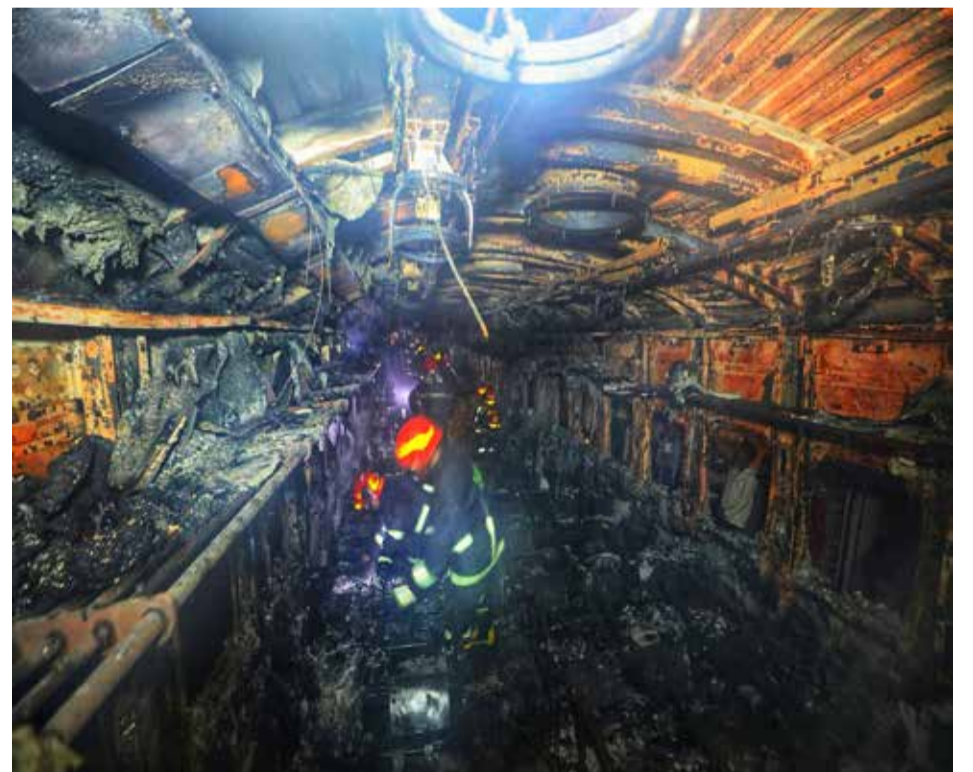
DHAKA: Bangladeshi fire fighters search through a burnt out carriage of the Benapole Express in Dhaka on January 5, 2024. — AFP
