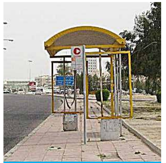
Poorly maintained bus-stop.
