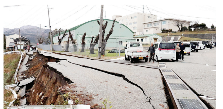
WAJIMA, Japan: People stand next to large cracks in the pavement after evacuating into a street on Jan 1, 2024 after a major earthquake struck the Noto region in Ishikawa prefecture. — AFP
