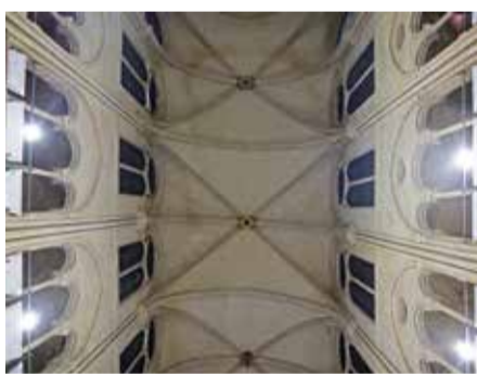
This photograph shows the vault of the nave of the Notre-Dame de Paris Cathedral, during its reconstruction after the fire that destroyed the Cathedral April 15, 2019.
