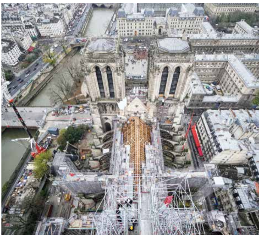
This photograph taken from atop the Notre-Dame de Paris Cathedral shows the structure of the building during reconstruction work, on the Ile de la Cite in Paris.
