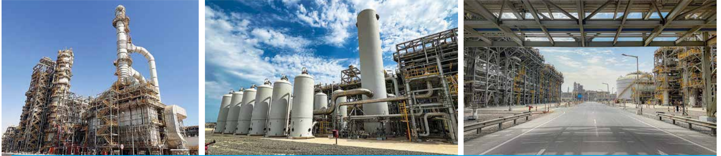
KUWAIT: Photos show the Al-Zour refinery. The Kuwait Integrated Petroleum Industries Company (KIPIC) announced on Sunday the successful and safe completion of the operation of the third and final units of the Al-Zour refinery. — KUNA photos
