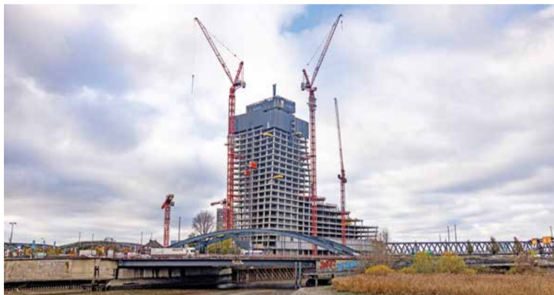
HAMBURG: Picture taken in Hamburg, northern Germany, shows the suspended construction site of the Elbtower, a project by Signa group, that was expected to be one of Germany's tallest buildings and was halted at the end of October 2023. -- AFP
