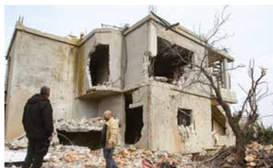
AITAROUN: Lebanese farmer and minibus driver Abdallah Abdallah (left) inspects his damaged home on Nov 25, 2023. — AFP
