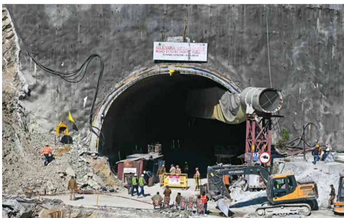
UTTARKASHI, India: Rescue personnel work at the mouth of the collapsed under construction Silkyara tunnel in the Uttarkashi district of India's Uttarakhand state, on November 24, 2023. - AFP
