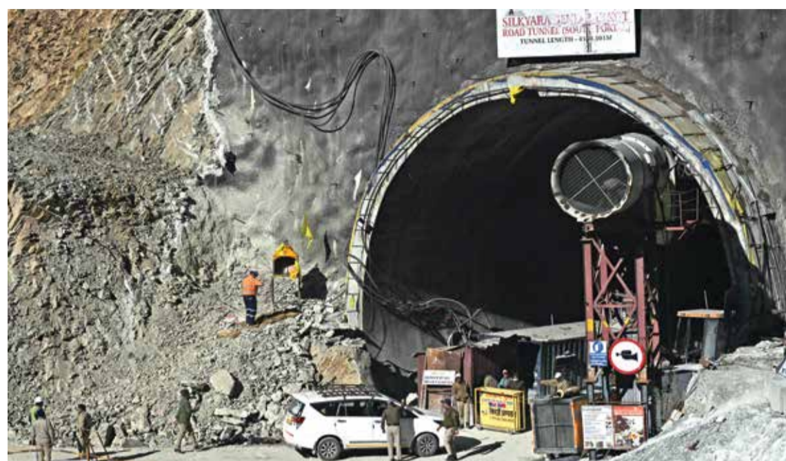
UTTARKASHI: A general view shows the entrance of the under construction Silkyara road tunnel during rescue efforts for trapped workers. — AFP photos
