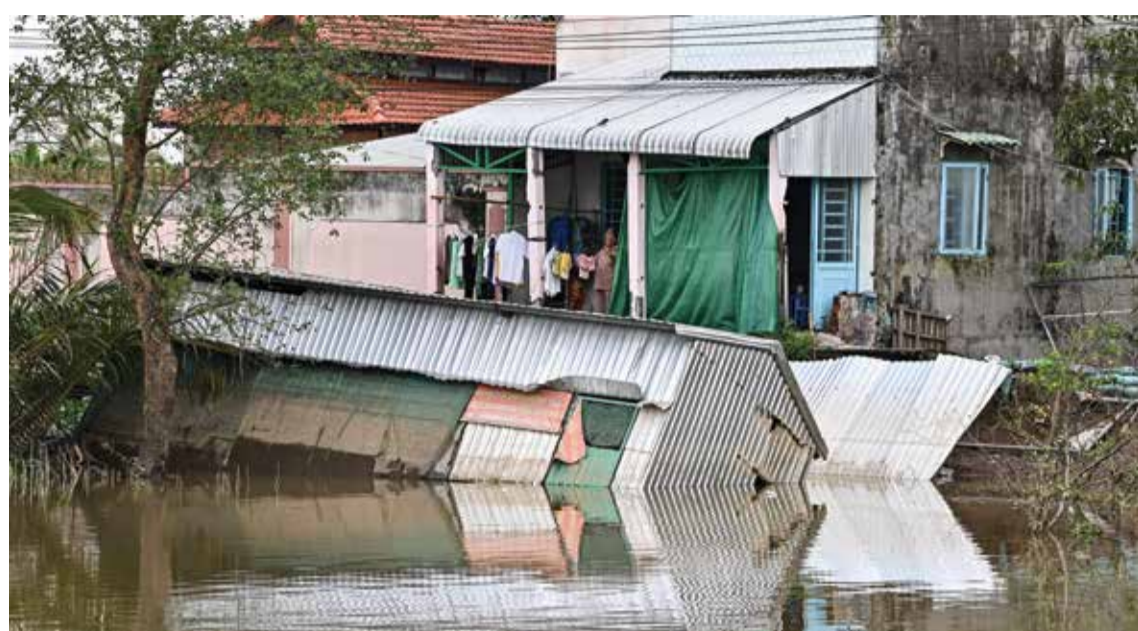
CAN THO, Vietnam: This photo taken on October 26, 2023 shows the site where resident Le Thi Hong Mai's house collapsed into the Hau river due to erosion in Can Tho city in southern Vietnam. — AFP
