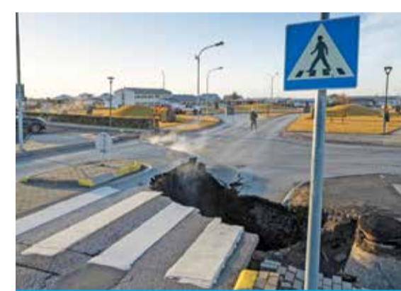
GRINDAVIK: This photo taken on Nov 13, 2023 shows a crack cutting across the main road in Grindavik, southwestern Iceland following earthquakes. — AFP
