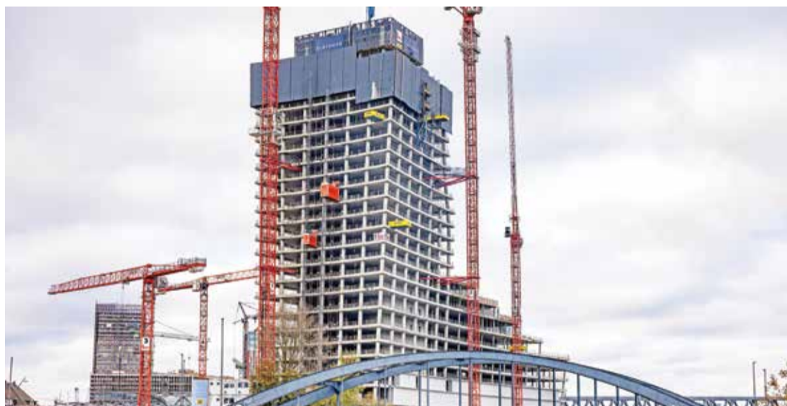
HAMBURG: Picture taken on November 16, 2023 in Hamburg, northern Germany, shows the suspended construction site of the Elbtower, a project by Signa group, that was expected to be one of Germany's tallest buildings and was halted at the end of last October 2023. -- AFP
