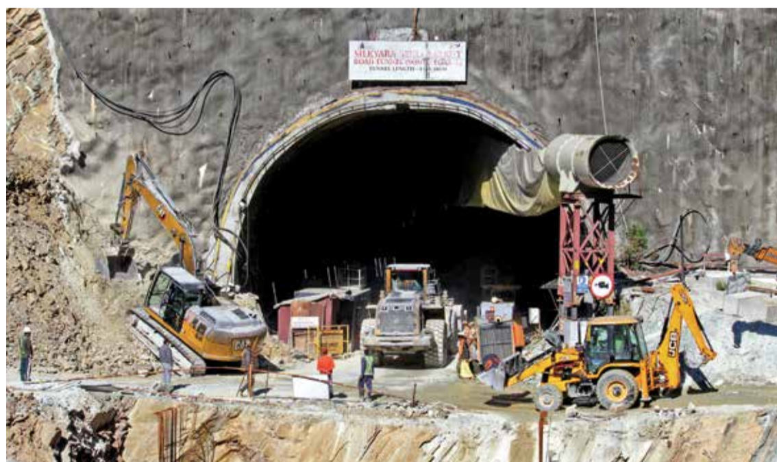
UTTARKASHI: Rescue workers stand at an entrance of the under construction road tunnel on Nov 18, 2023, days after it collapsed. — AFP
