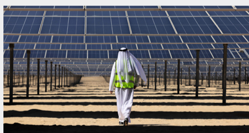
An Emirati man walks beneath photovoltaic panels at Al Dhafra Solar PV IPP project on Nov 13, 2023. — AFP
