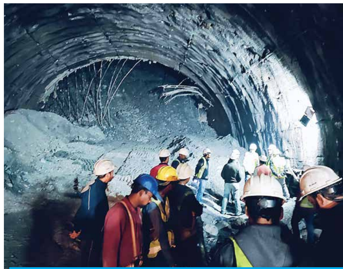
UTTARKASHI: In this photograph taken on Nov 12, 2023, rescue workers gather at the site after a tunnel collapsed in the Uttarkashi district of India's Uttarakhand state. — AFP
